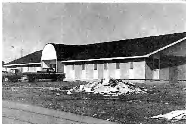
TO YOUR HEALTH — The new Pleasant Point Health Center will be occupied by mid-April and dedicated in early May. The $225,000 complex was started last October. It is owned by the tribe and will be leased to Indian Health Services. The lease will be negotiated this month.
