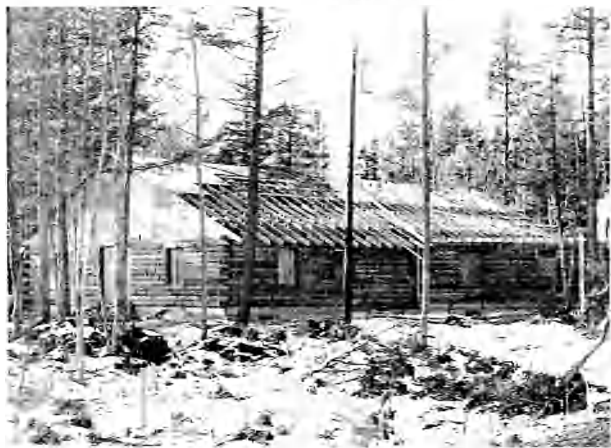
RUSTIC STRUCTURE —This log style, Y-shaped building at Indian Island will eventually house an early childhood program for the school, and a Penobscot tribal museum. The Young Adult Conservation Corps [YACC] is assisting in construction.
