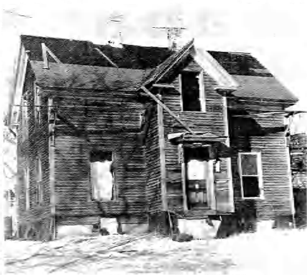
DERELICT — Once a handsome dwelling at Indian Island, this twin-chimney house has been left vacant — except for young people who now use it as their "hangout" after school. This home boasted the first running water on the reservation, and was known for its hardwood floors. Several old treaties were discovered in this house years ago. They were sold to the Bangor Public Library, but later recovered by the Penobscot tribe.
